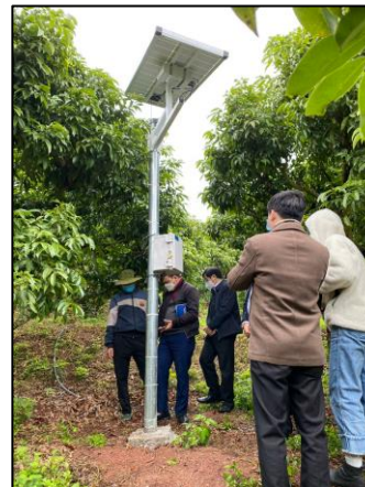
Installing sensor stations to improve quality of lychee and productivity in Viet Nam
